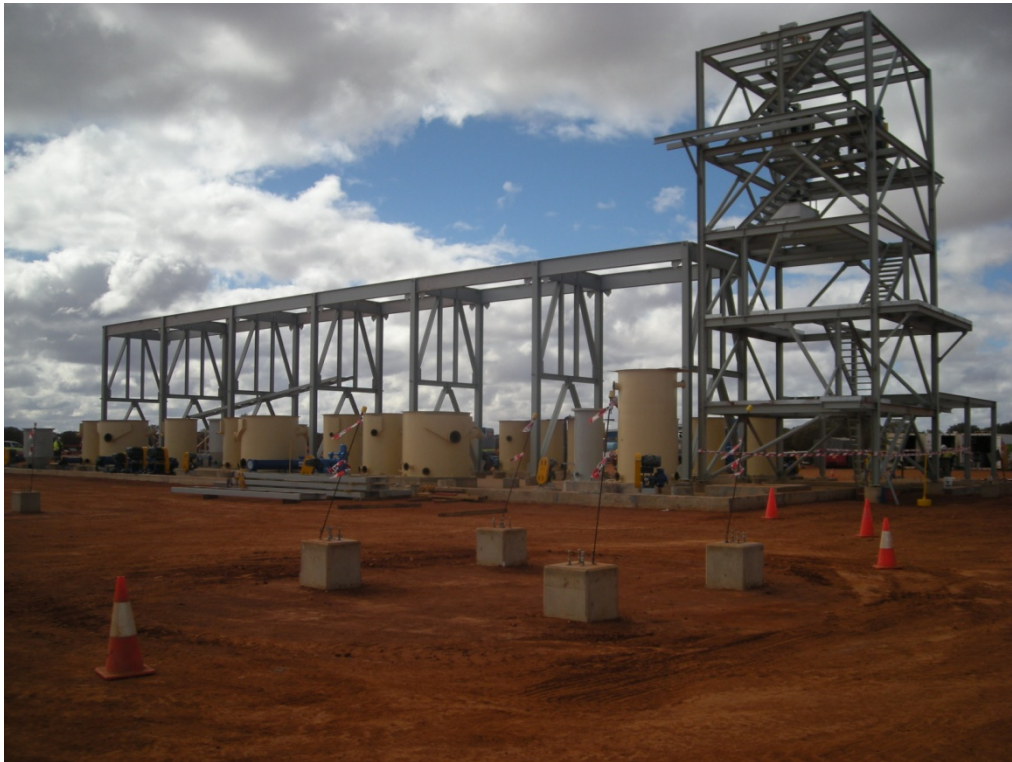
Steelworks erected above the flotation building at the Concentration Plant, Western Australia
